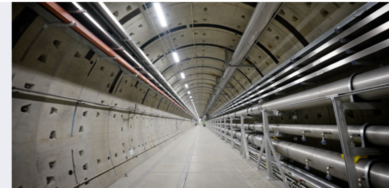
Inside the underground tunnel of the SHINE facility.
